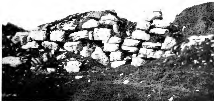
FIGURE 5. — A PIECE OF THE OUTER WALL ON THE WEST SIDE South of point 9
